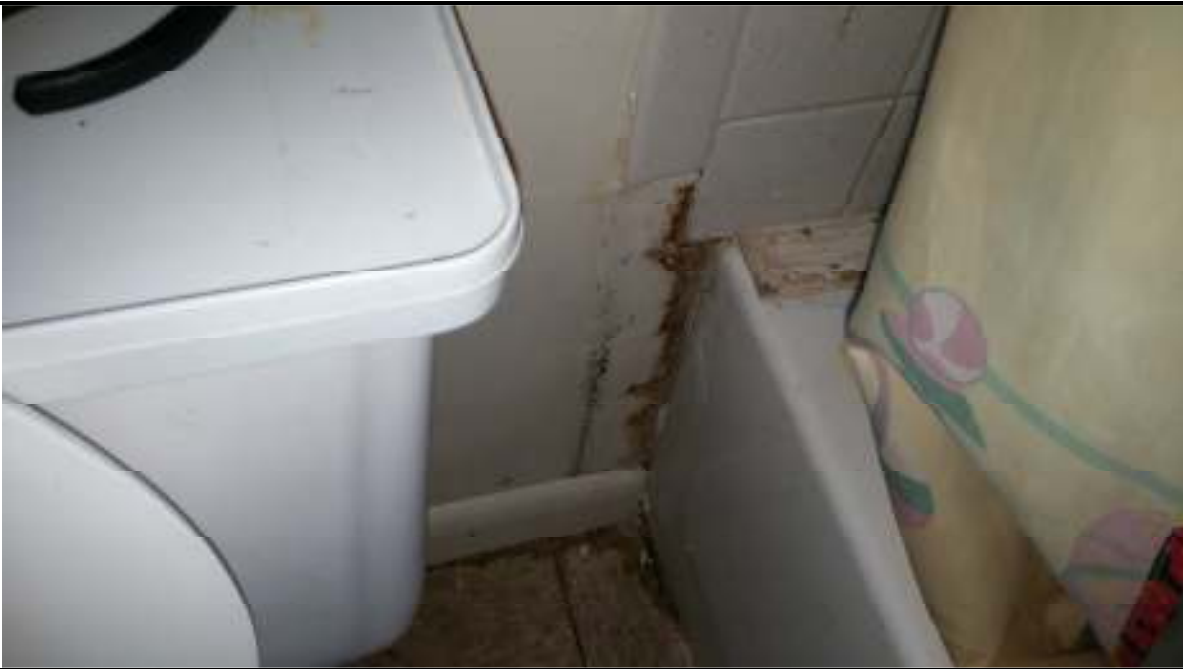
Photo 9: Visible mold growth inside of the restroom in Unit 70.
