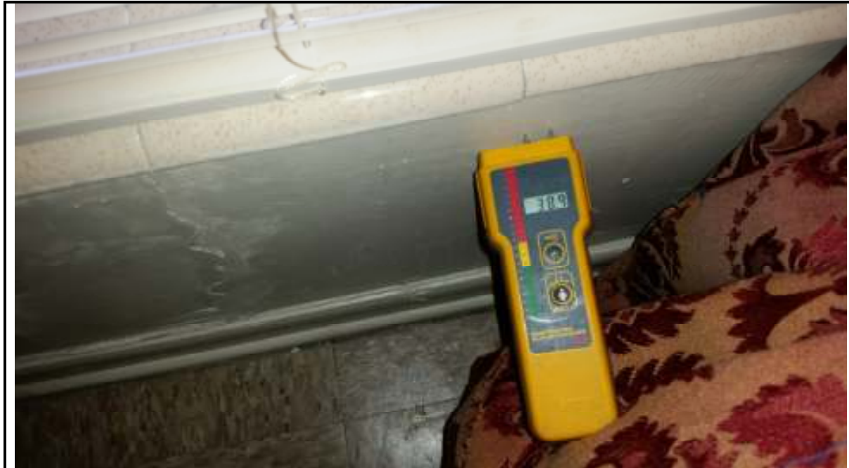
Photo 5: Typical elevated moisture meter reading.
