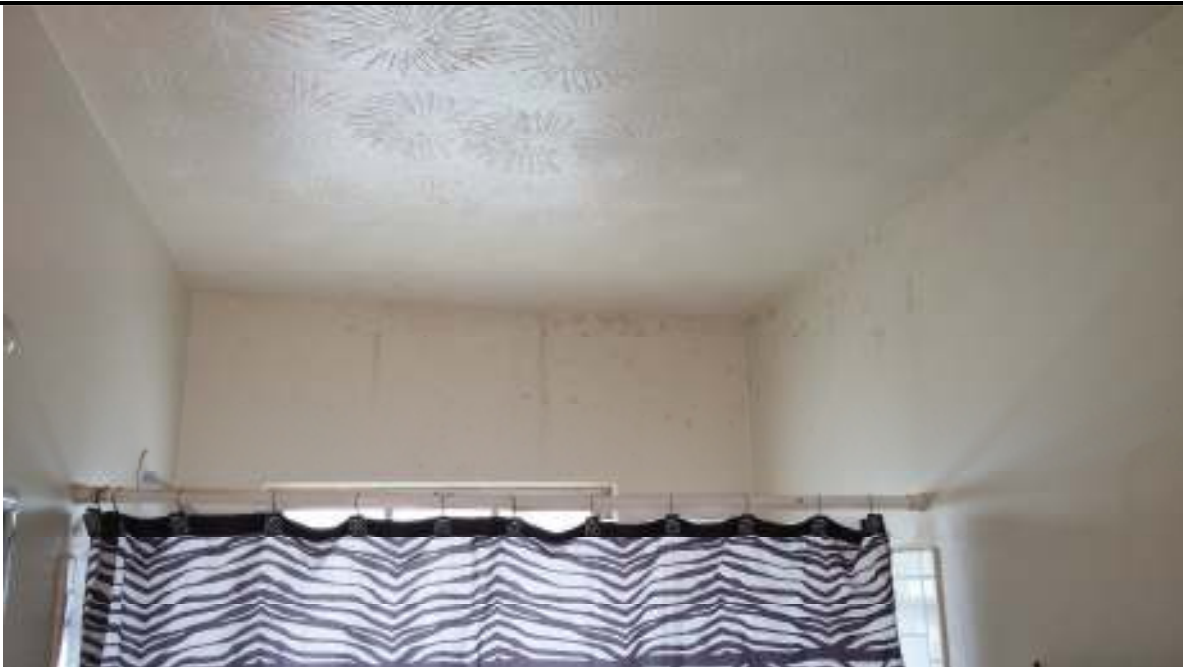
Photo 7: Visible mold growth inside of the restroom in Unit 364.
