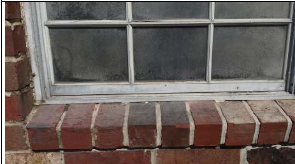
Photo 6: Typical condition of deteriorated caulking on the outside of the windows.
