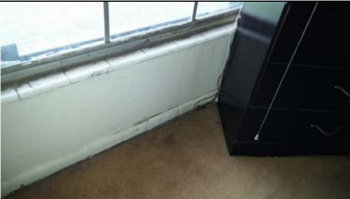
Photo 10: Visible mold growth inside of Unit 226 below livingroom window.
