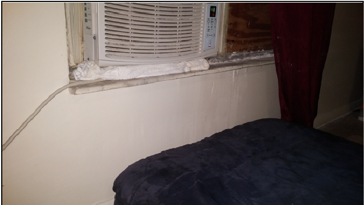
Photo 1: Typical water damage and wall repairs beneath windows.
