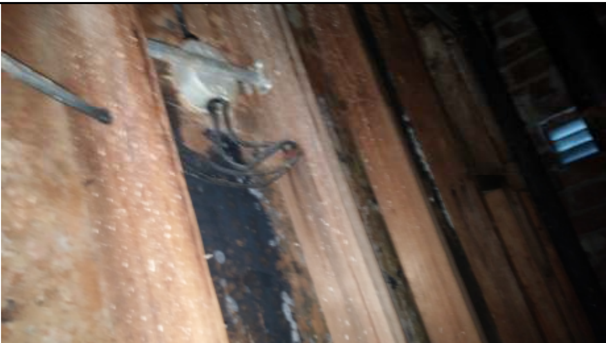
Photo 12: Visible mold growth inside of Unit 265.
