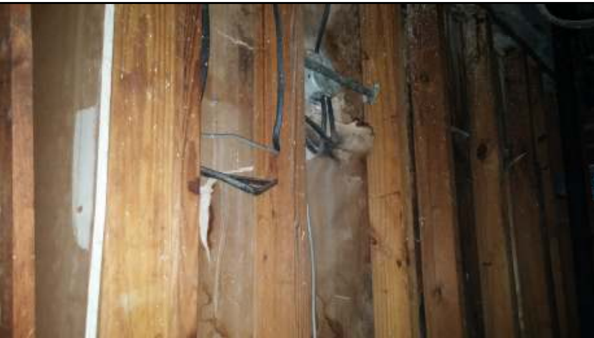
Photo 8: Visible mold growth inside of Unit 376.
