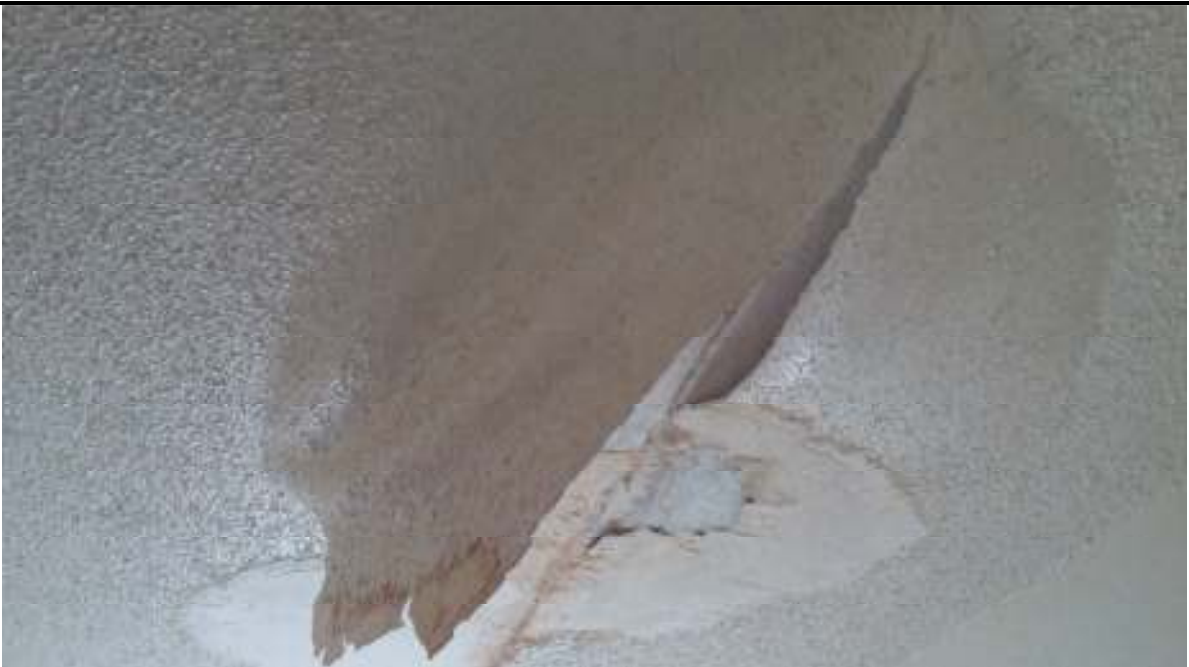
Photo 11: Ceiling damage due to water intrusion in the restroom in Unit 265.
