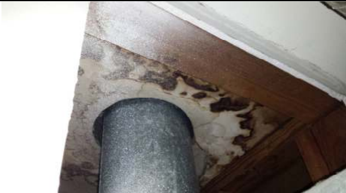
Photo 4: Visible mold located in Building 15, Unit 150.
